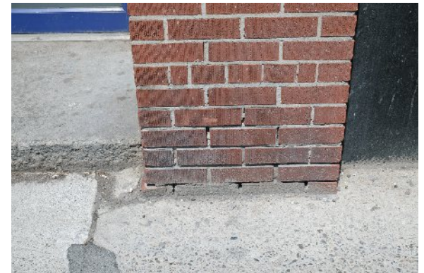
38. Detail of eroded joints near the base of the S. wall from rising damp and deicing salts. PGA
