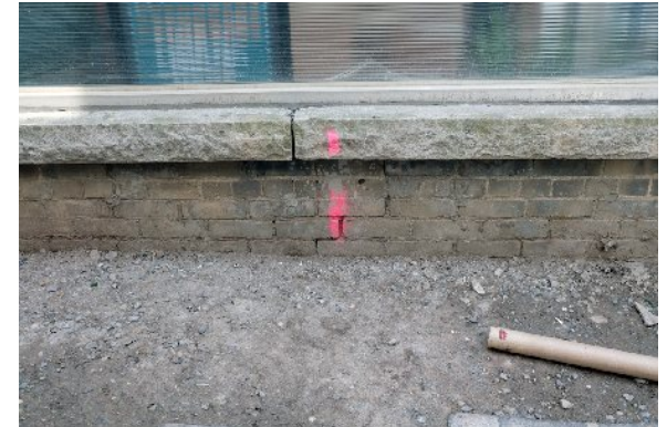
40. Detail of eroded joints near the base of the n. wall. PGA
